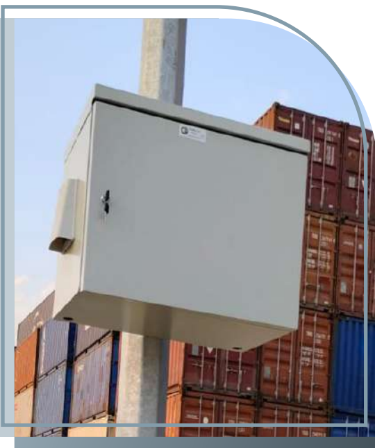
OUTDOOR CABINETS POLE/WALL TYPE
